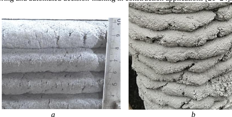
Figure 1 - Layer delamination & surface texture
